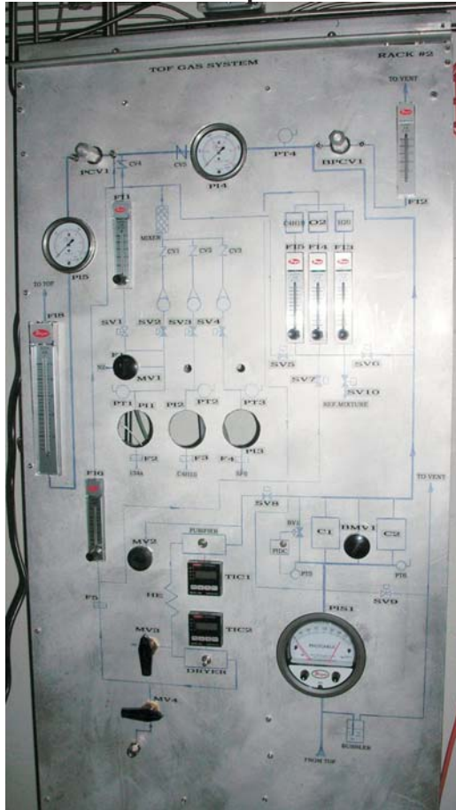
main control panel
