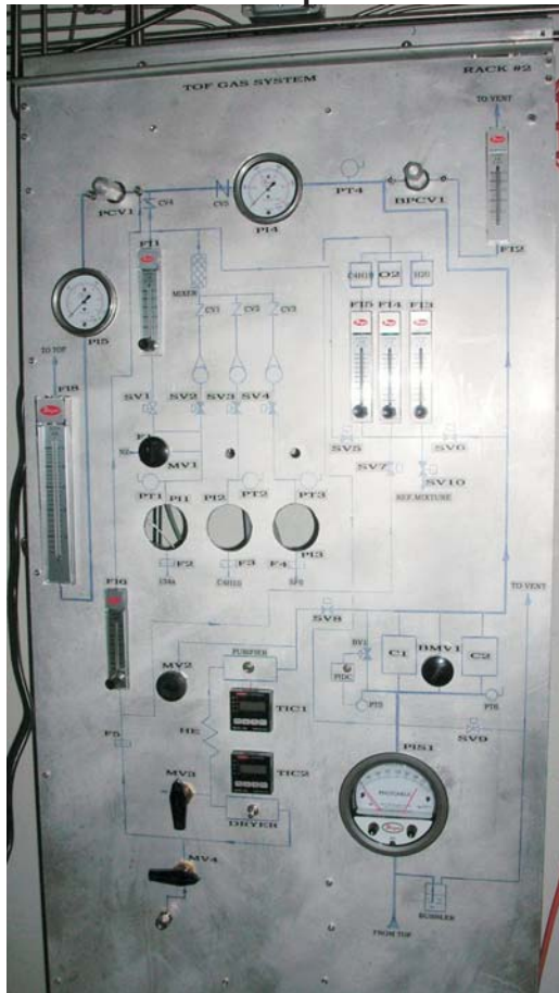
main control panel
